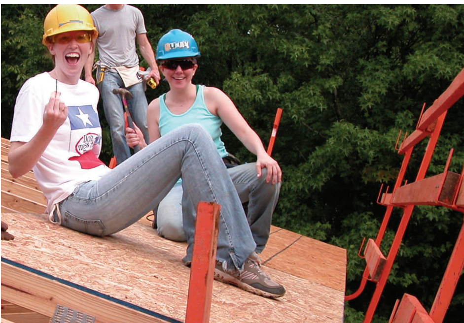
On top of the world. Sheena Bossie and Susan Pierson (left) show how it's done when it comes to installing plywood on the soon-to-be completed roof.
