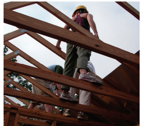
Volunteers walk a wooden tightrope as they finish the roof. Hardhats and safety glasses are musts for volunteer workers.
