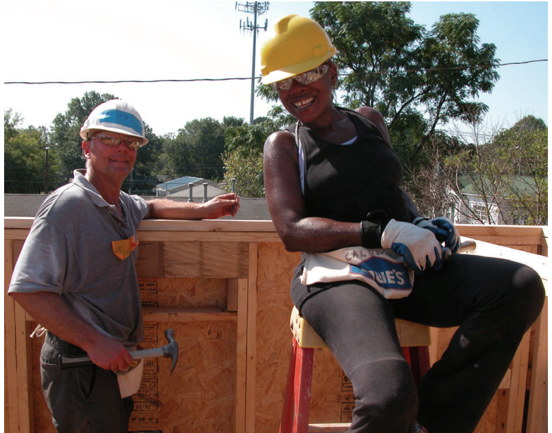
As is the custom of many members, nearly 10 Caldwell volunteers rolled up their sleeves on a broiling hot Saturday to help frame a home for Habitat for Humanity on Charlotte's west side. Jim Curtis shows new member Zoraida Stewart the fine points of wielding a hammer. After watching Yvette deftly pound nails, it's evident she will be passing out coaching advice soon enough.
