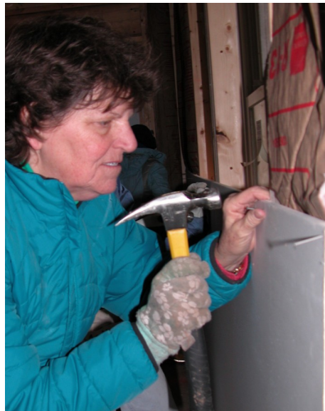
Joyce Deaton sets a nail with a few well aimed smacks. The sheet was then lifted into place. A few whacks later and the nail - and the sheet of drywall - was firmly in place.
