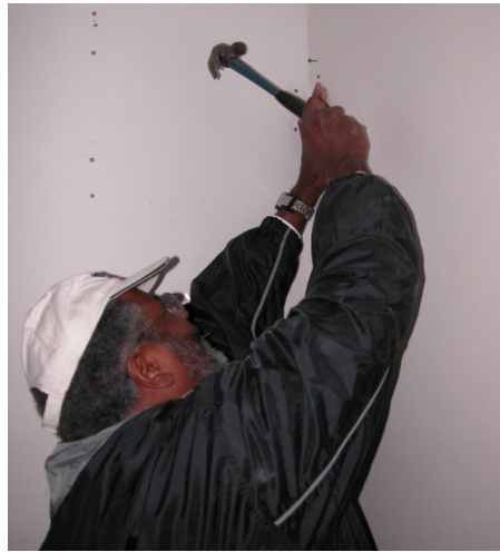
Like a seasoned pro: John Chandler deftly wields a hammer (it doesn't hurt to be tall) to drive nails high on an interior wall.
